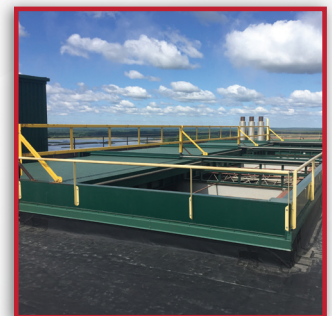
Sliding Roof Hatch
