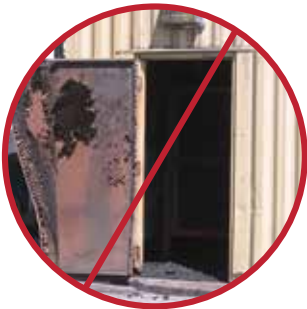
Failed Hollow Metal Door
